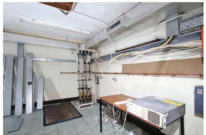
The PMBX room with a small MDF. The Compaq unit on the table is an old PC/server
